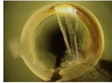
Picture above: Likely illicit sump pump connection discharging inflow of clear water into the sanitary sewer. NEW Water Televising Program 9/6/2018.
