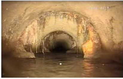
Picture above: Root intrusion into a pipe indicates likely infiltration of clear water and can block sewer flow. NEW Water Televising Program.
